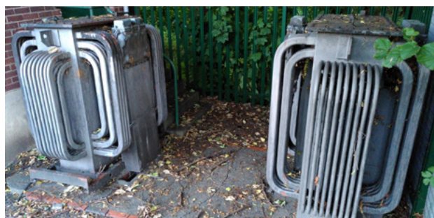
Aging transformers need to be replaced with smart infrastructure.
